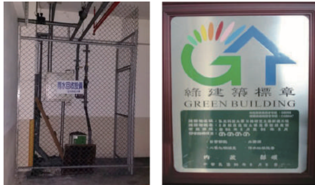
Fig. 5-8 Rainwater recycling system complied with Green Mark
